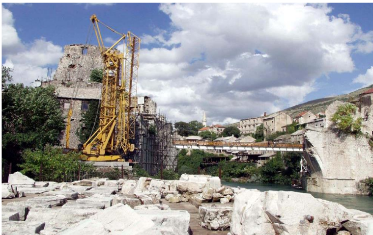
Picture 8: The start of reconstruction of the Old Bridge, mounting of the first crane and scattered stone blocks on the platform by the river
