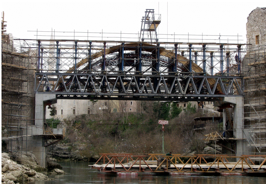
Picture 12: Arch scaffolding on the concrete foundations with the pontoon bridge over the Neretva river
